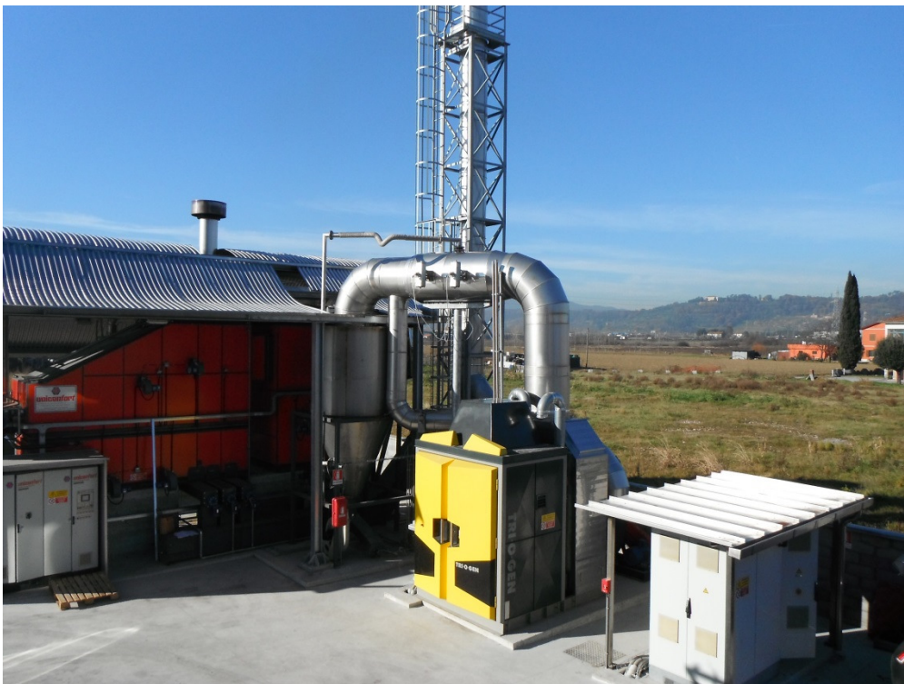
Figure 3: Example of a biomass fired ORC plant
