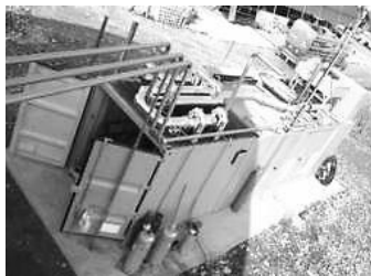
Figure 7: Treviso ORC container with exhaust heat recovery
