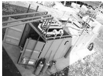
Figure 7: Treviso ORC container with exhaust heat recovery
