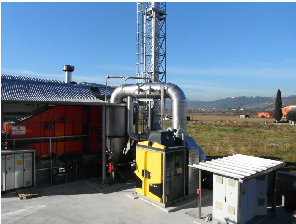
Figure 3: Example of a biomass fired ORC plant
