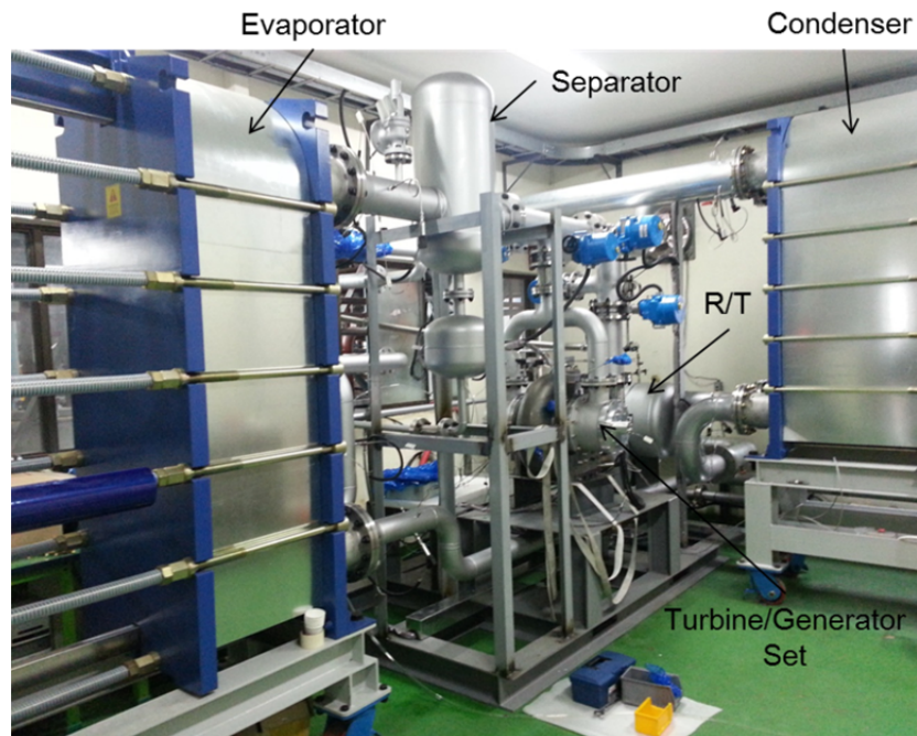
Figure 6: Photo of a 100kW Geothermal ORC Turbo-generator
