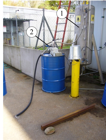
Figure 9: New vacuum pump fluid reservoir and membrane pump
